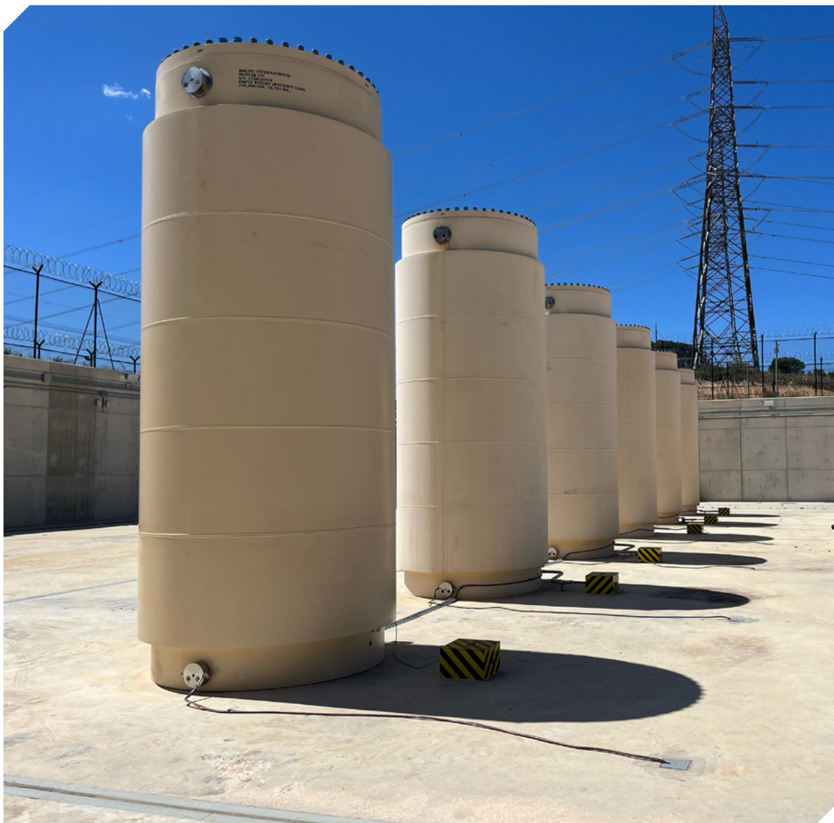
General view of the Cofrentes Nuclear Power Plant ITS.
